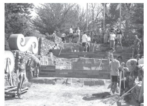
Dozens of volunteers dig out the dirt and build tiers for plantings.
